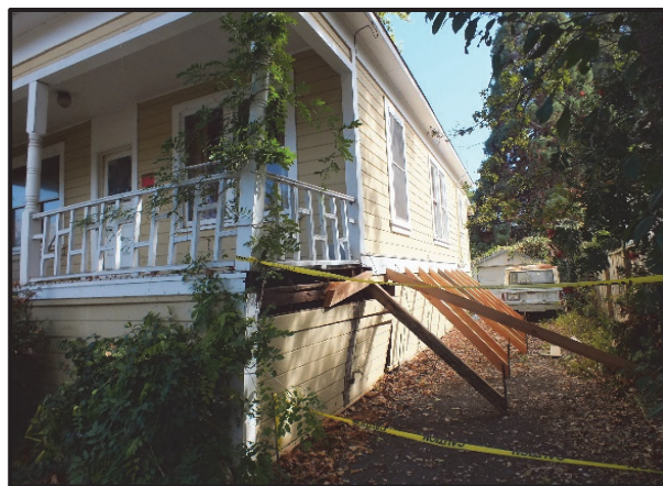
Figure 1: House with cripple walls damaged in the South Napa earthquake. Temporary bracing has been installed to provide stability and prevent collapse. Photo credit: Estructure.
