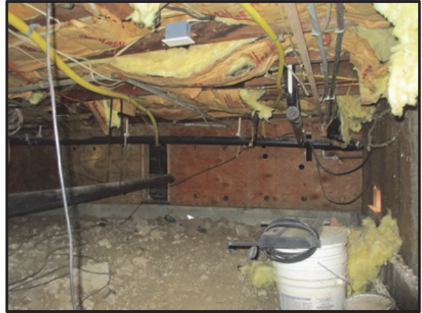
Figure 2: Cripple wall with plywood strengthening that was undamaged in the South Napa earthquake. Photo credit: ZFA Structural Engineers.
