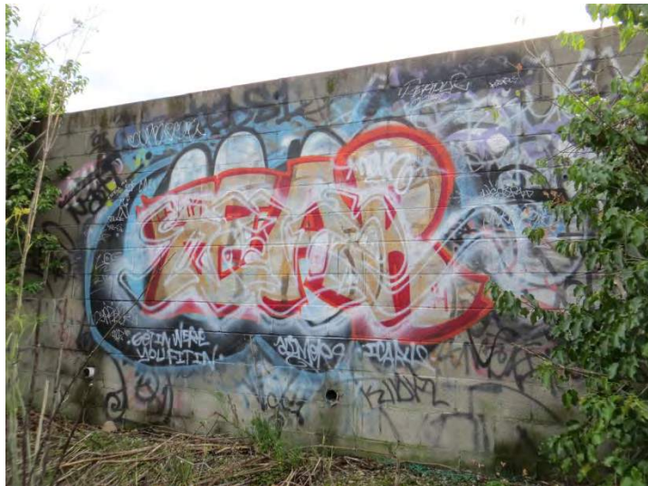
Graffiti along Americorps Trail, on wall of old concrete plant.
